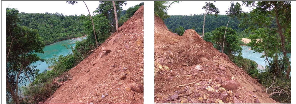
Dumping near powerhouse adjacent to the river Kopili
